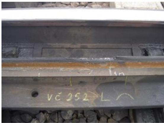
Figure 62 – Crumbled switch rail
