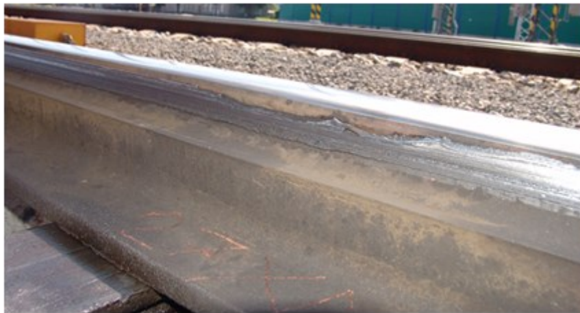
Figure 40 – Switch rail crumbling
