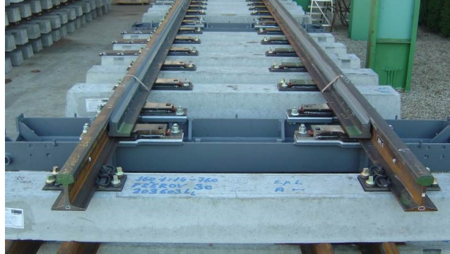
Figure 21 - Switch panel on concrete sleepers
