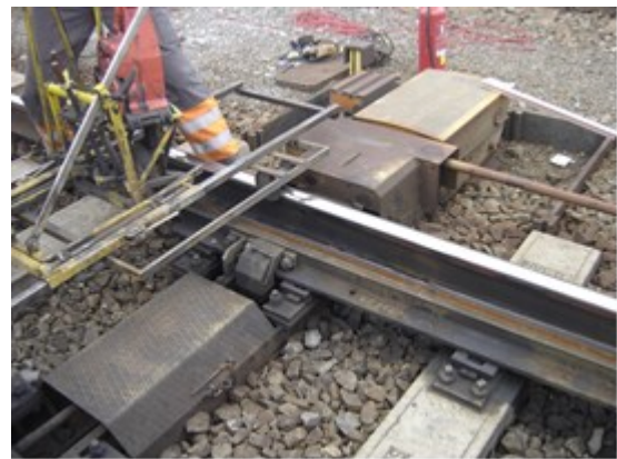
Figure 63 – Crumbled switch rail before grinding
