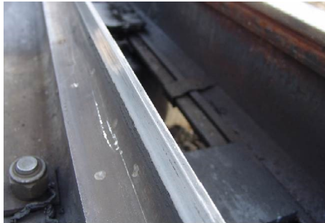
Figure 39 – Lateral degradation of the switch rail tip with the wheel's running profile
